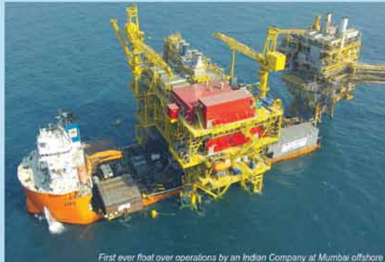
First ever float over operations by an Indian Company at Mumbai offshore
